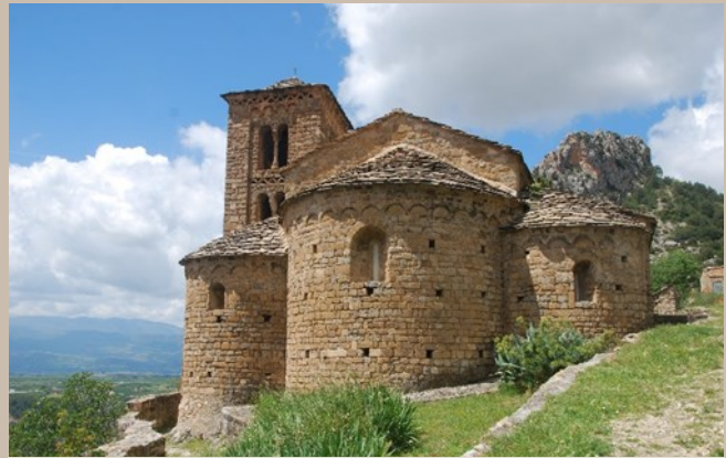
Sant Esteve church (built in 1141 and used into the 1980's) in the village of Abella de la Conca.
